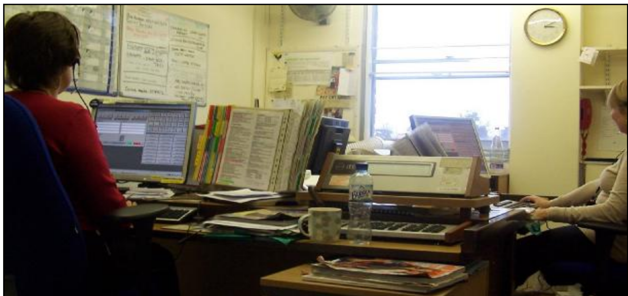
EFDC's switchboard is housed in a small room on the first floor of the Civic Offices
